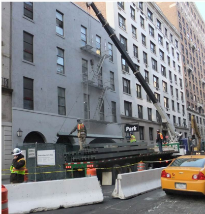
Ancillary 1 - Structural Steel Delivery on 63rd Street between Lexington and Park Aves
