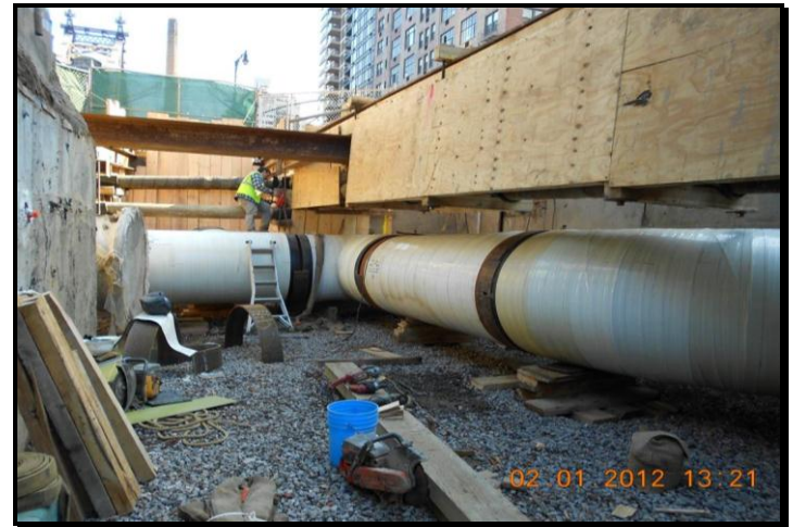
Installation of the 48-inch trunk water main on E. 59 th St. between 1 st Avenue and 2 nd Avenue
