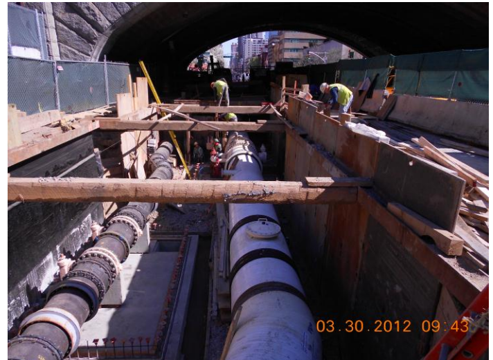
Workers installing 48" trunk water main and 24" piping for the pressure regulator valve on 1 st Ave. between E. 59 th St. and E. 60 th St.
