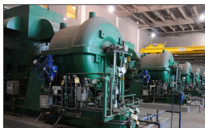
Blower at the Newtown Creek plant
