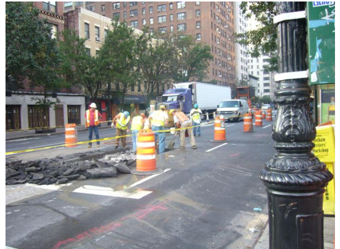
Workers perform 20-inch gas main relocation on 1 st Ave. between E. 58 th St. and E. 59 th St.
